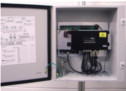
FIGURE 2. The CMM4 Includes 14 Port Ethernet Switch, GPS Antenna and Cables
